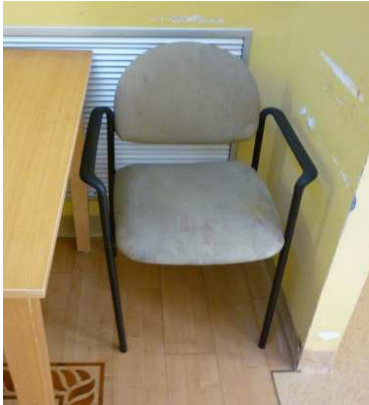
Image 8: Soiled Chair and damaged wall.
